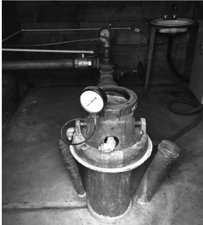
Figure 5: Image of the well pump for Well #2.
