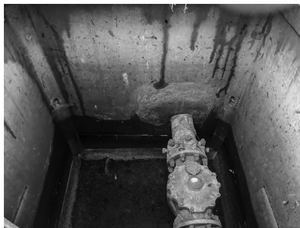
Figure 12: Image of vault. Note the bowing around the pipe grout. The grout itself was not installed to appear bowed, bowing is due to hydrostatic pressures pushing against the vault.
