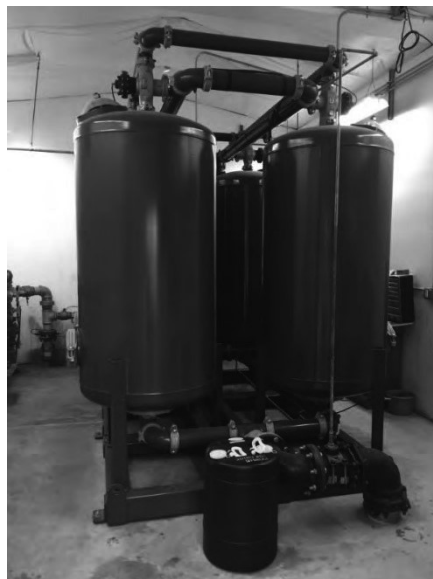
Figure 8: Image of arsenic treatment apparatus at Well #1.
