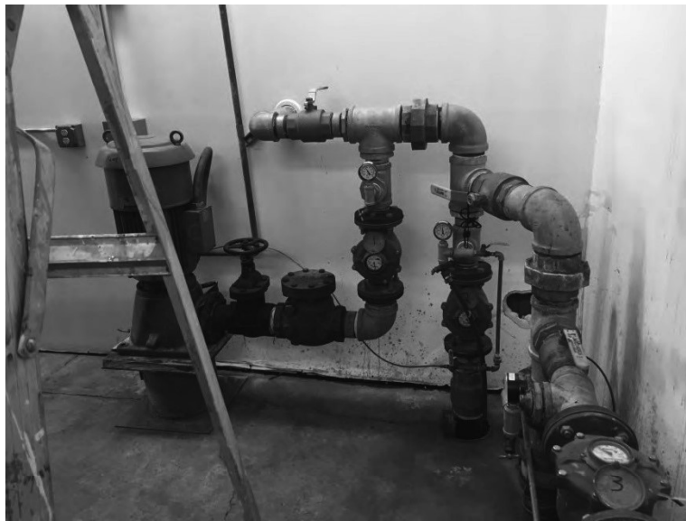
Figure 4: Image of the well pump for Well #1.
