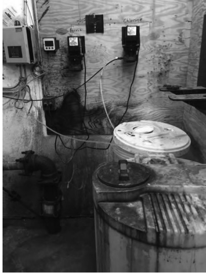
Figure 9: Image of chlorine injection system at Well #1.
