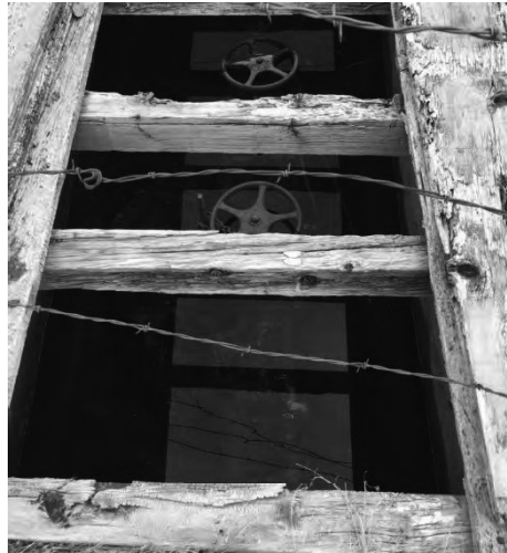
Figure 11: Image of inside the vault at the Forest Service outpost filled with groundwater. Note the level of encrustation visible on megalugs and flanges.
