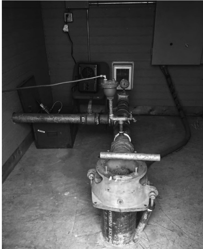
Figure 6: Image of the well pump for Well #3.
