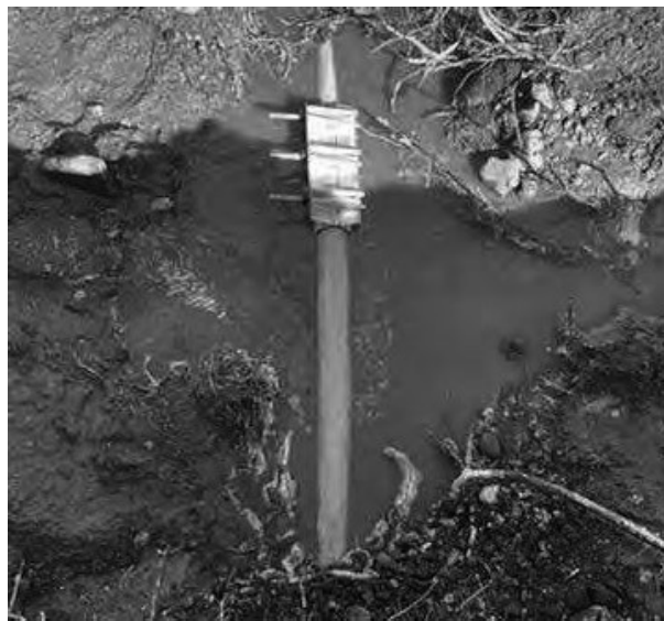
Figure 10: Image of a leak discovered in the distribution system where pipe has been exposed to fix the leak.
